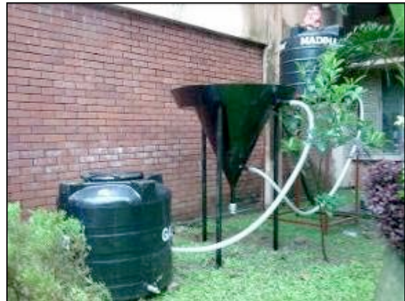
Photo: Four hundred liter prototype water treatment system consisting of a mixing tank, clarifier, and storage tank, which is temporarily installed at BUET for testing. Photo credit: Mahbuba Iasmin Ahmed (July 2008)
